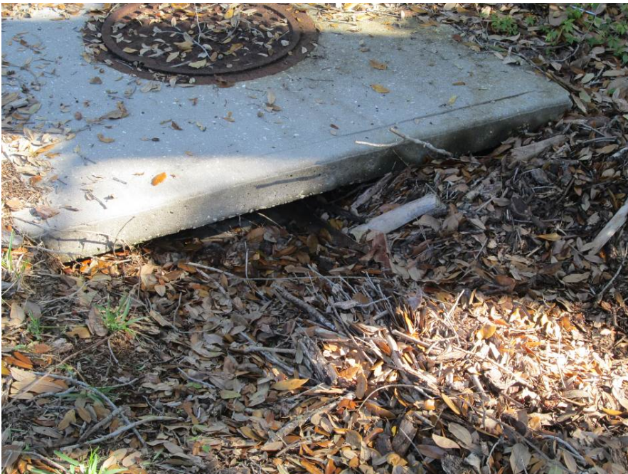
Leaves and debris in front of throat inlet at Dry Retention Pond
